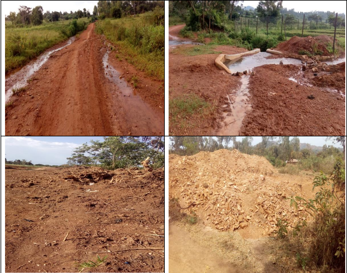
Plate 4.1: Watershed destruction activities due to County roads infrastructure in the Lower Sio River Basin
