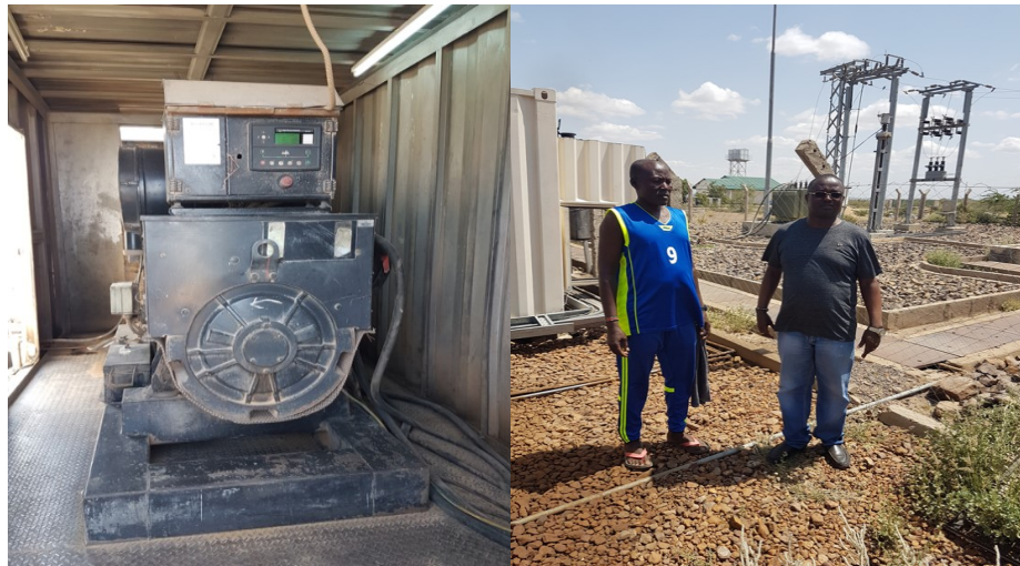
Plate 6.3 500 KVA diesel generator that supplies Kakuma Town and Environs.
