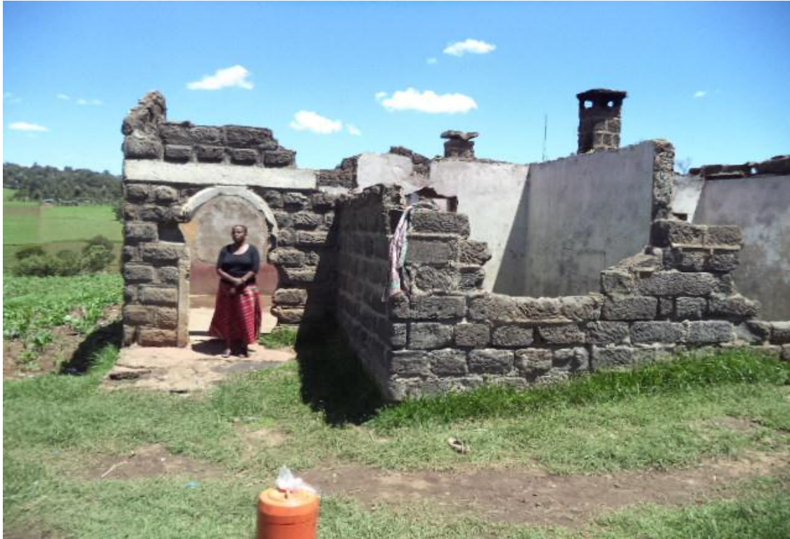
Plate 6: The researcher walking out of the remains of a house in Sachangwan that belonged to Kagiri that had been burnt down during the 2007/8 post-election violence
