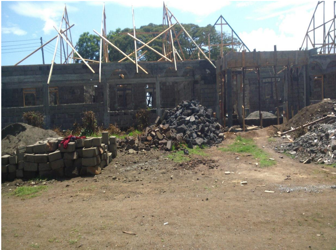
Plate 8: A hotel in Githima, Nakuru, being constructed after having been burnt down in 2007/8 post-election violence
