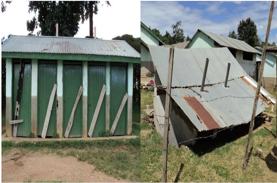
Plate 1: Collapsed pit latrines in at Bishop Sulumeti Girls (Kakamega Central)
