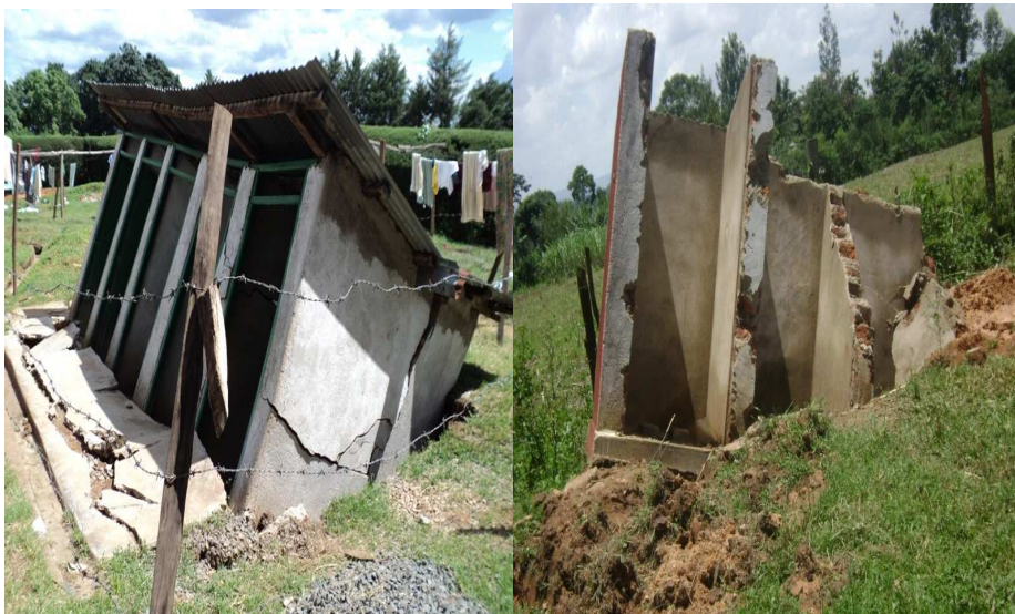
Plate 2: Collapsed pit latrines-Bishop Sulumeti Girls (Kakamega Central) & Chiliva Primary School (Kakamega North)
