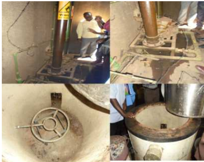
Plate 20: Removal of sulphur traces before delivering gas to the kitchen
