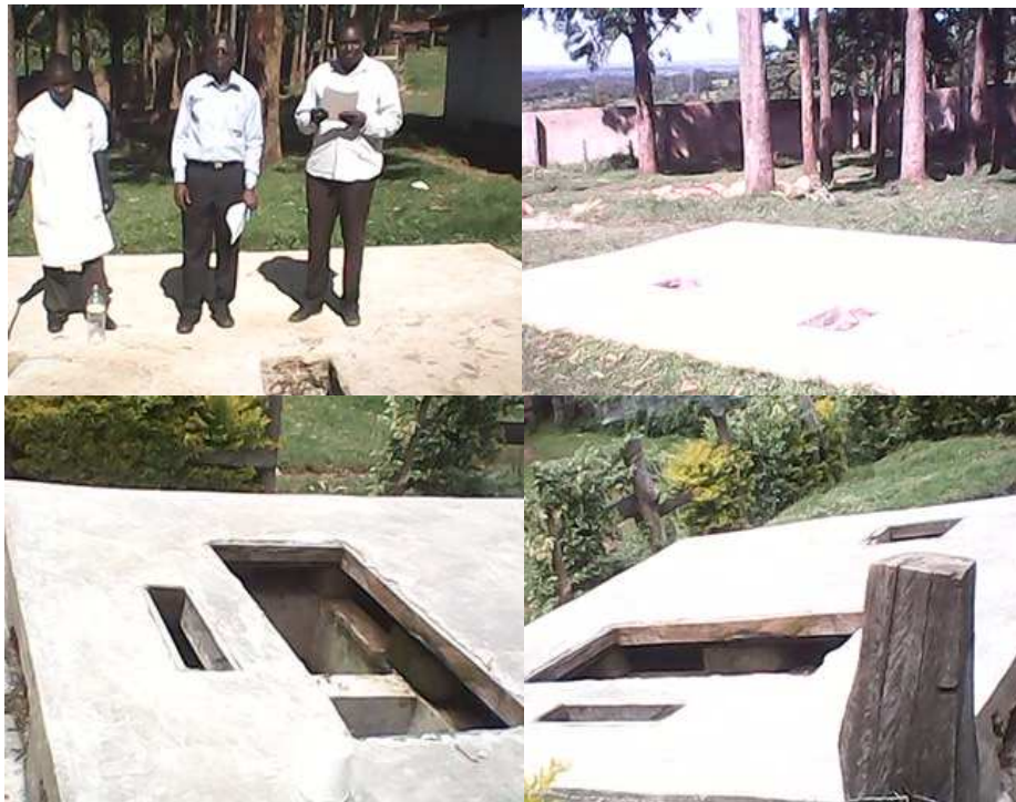
Plate 4: Open manholes in some of the schools
