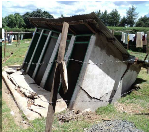
Plate 4.3b: Collapsed pit latrines
