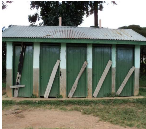
Plate 4. 3a: Condemned pit latrines
