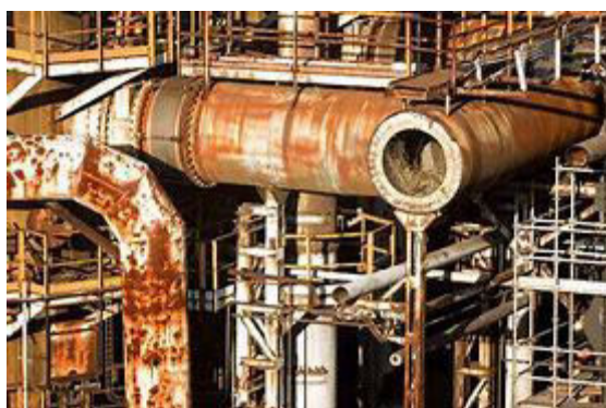
Figure 1-2-Effect of fly ash corrosion on industrial equipment (Source: Mumias Sugar company, 2013)
