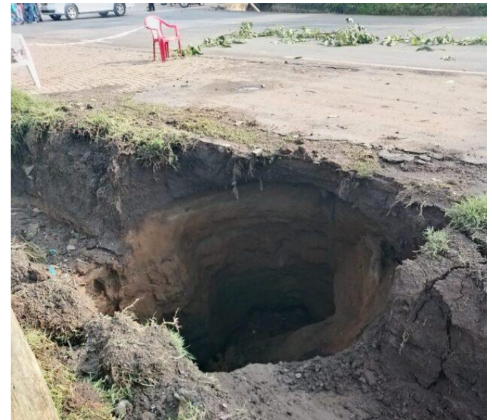
The sinkhole is on the road side at National Filling in London area of Nakuru Town West Sub-County.
