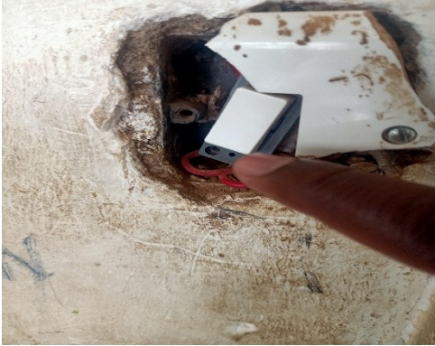
Plates 5.1: Electrical switch in a class
