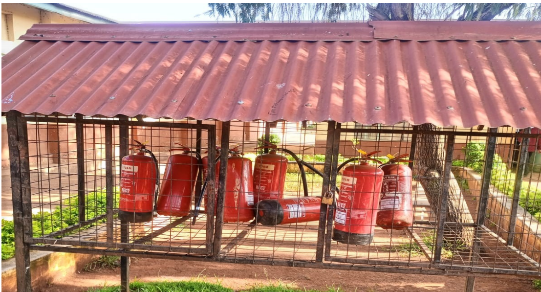
Plate 6.3 Showing few fire extinguishers locked in a cage
