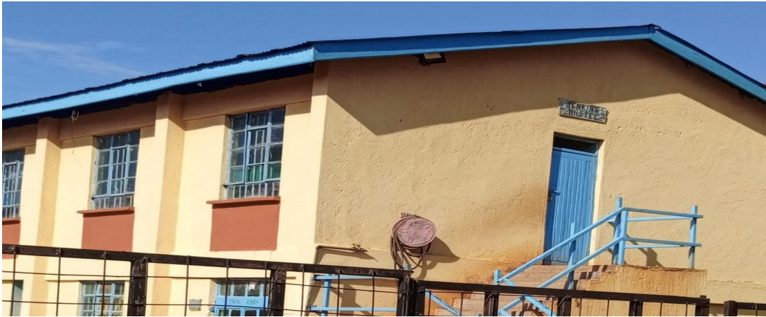
Plate 6.5 Mounted fire horse reel on a dormitory at Kimilili Boys.
