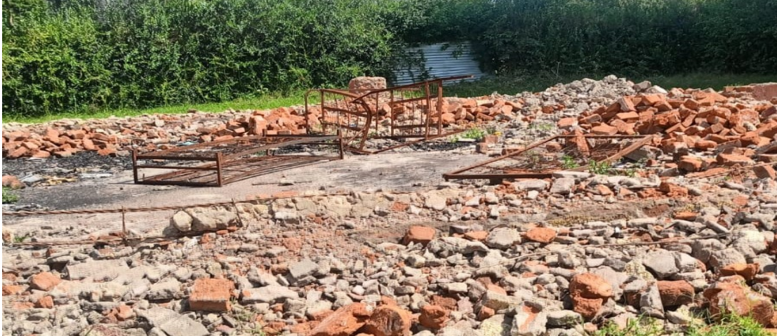
Plate 5.2 Showing remains of damaged students property
