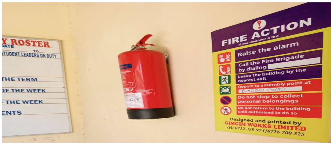
Plate 6.1 Fire extinguisher mounted with instructions at the office corridor
