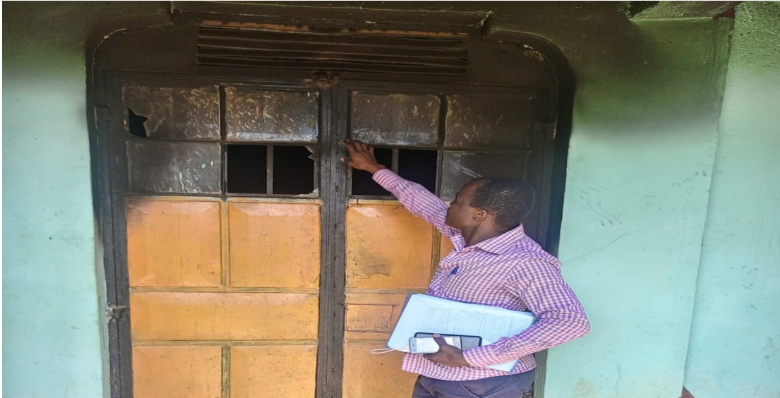
Plate 5.3 Research Assistant examining the impact of fire on a storey dormitory which has remained closed.
